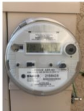
SMUD Electricity Meter
