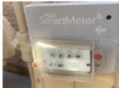
PG&E Gas Utility Meter
