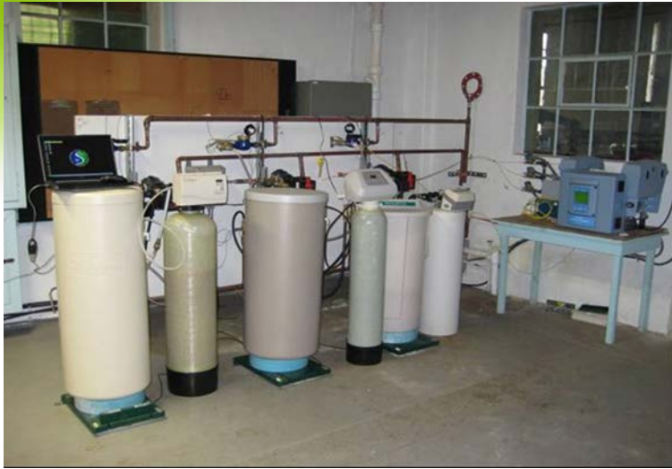
Waterloo test location, 36 gpg
