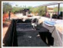
30,000 gallon underground cistern
