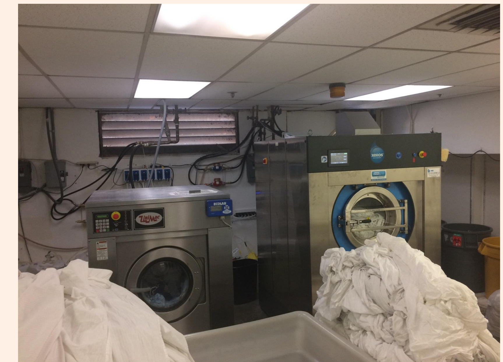
Conventional & bead technology 65-lb. washers in a hotel laundry facility
