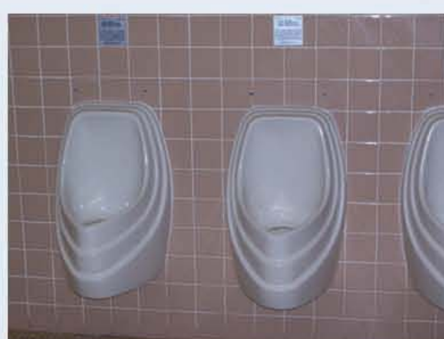
All urinals have been replaced with waterless urinals.
