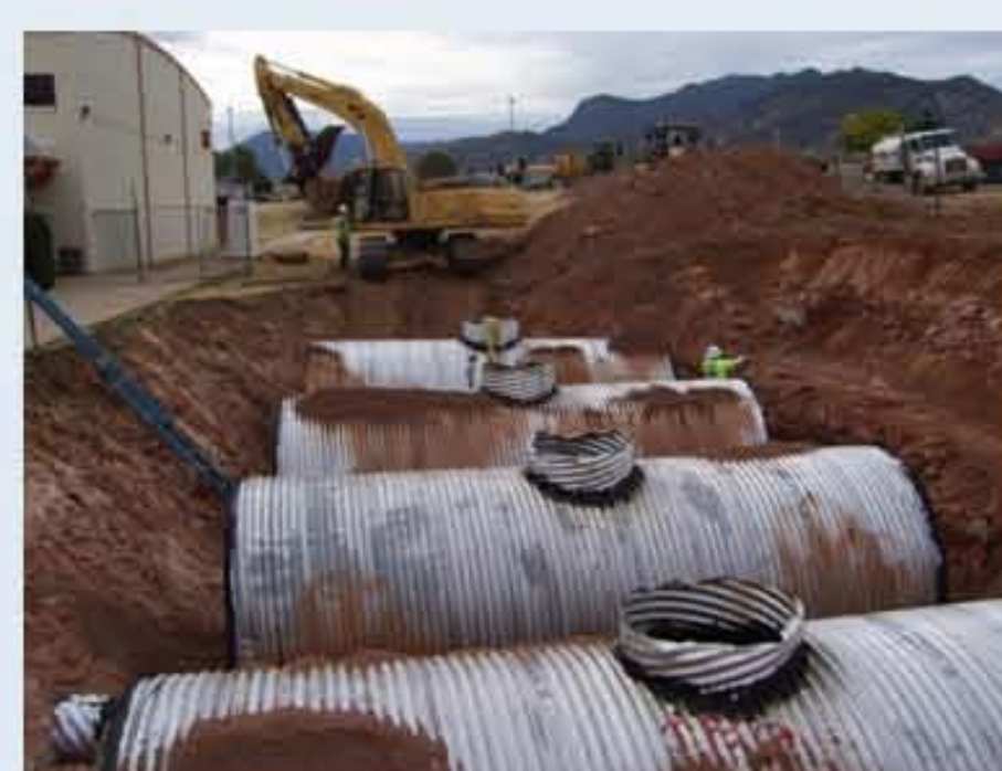
Rainwater harvesting and dry wells recharge the aquifer.
